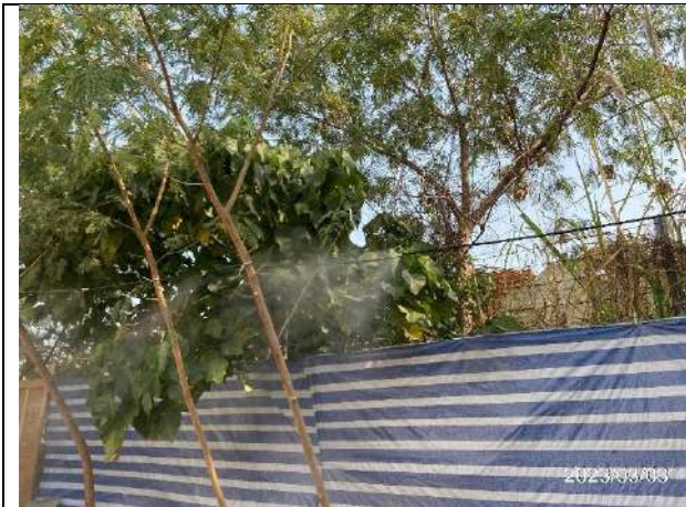
Photo 1: Organic Tech Ltd. Installed the odour suppression spray system at the northern boundary to minimize the odour impact.
