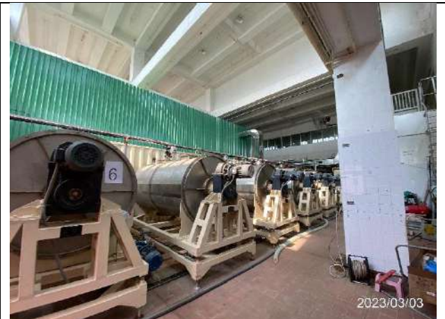
Photo 2: Slight odour of chicken manure smell was noticed in the works area of the chicken manure pre-treatment unit within the building.
