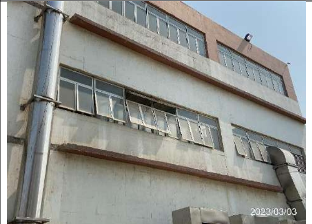
Photo 4: It is observed some of the windows of the building nearby the works area of the chicken manure pre-treatment unit were opening partially.
