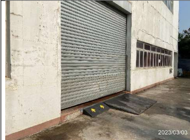
Photo 3: It is observed the roller shutter nearby the works area of the chicken manure pre-treatment unit was not fully enclosed
