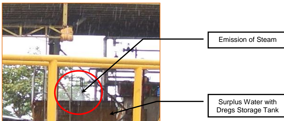
Photo 1 Steam emitted from gaps of the cover of the Surplus Water with Dregs Storage Tank
