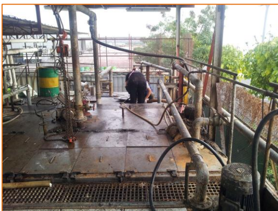
Photo 1 The top of the Oil/Water Mixture Storage Tanks and Surplus Water with Dregs Storage Tank
