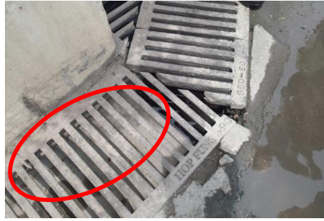
(Raised invert level observed on 16 May 2018)
