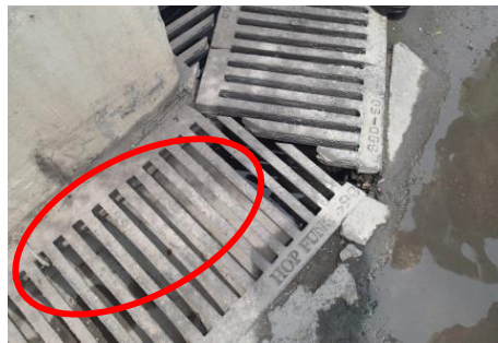
(Raised invert level observed on 16 May 2018)
