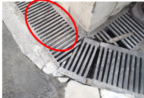
(Raised invert level observed on 20 June 2018)
