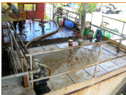
Photo 1 Covers of the Oil/Water Mixture Storage Tanks and Surplus Water with Dregs Storage Tank Remained Closed
