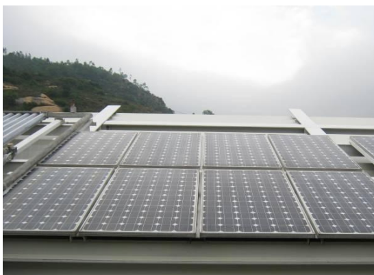
Solar Photovoltaic System
